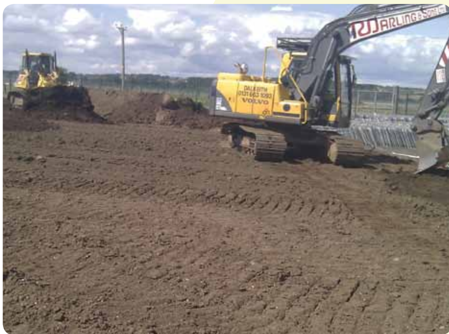
Work in progress. The area has already been seeded over and is showing encouraging growth.
